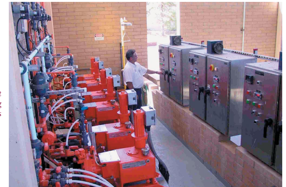
State certified treatment plant operator checking computer control panels
