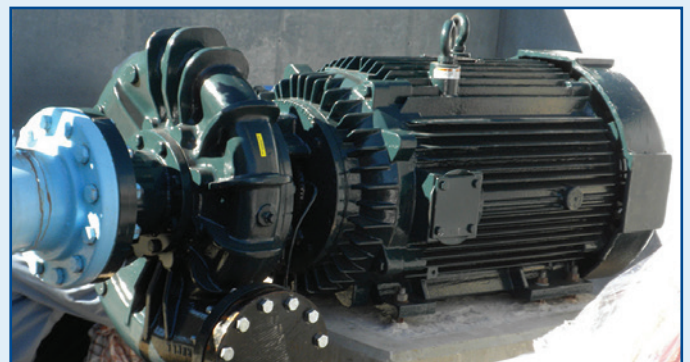
District pump station motor and turbine.
