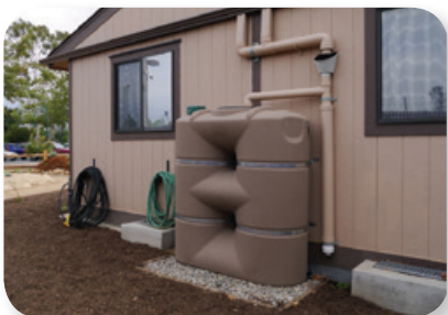
Rain Barrel Water Catchment System
